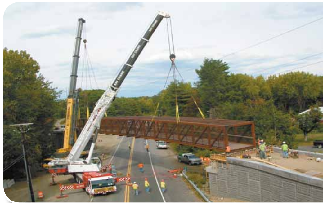
Locke Crane's Grove and Bay Crane's Link Belt place Continental Pedestrian Truss Bridge on Reinforced Earth supported abutments for E.T. & L. Corp.'s Northampton job. (All photos courtesy of Colton Andrews of E.T. & L. Corp.)
